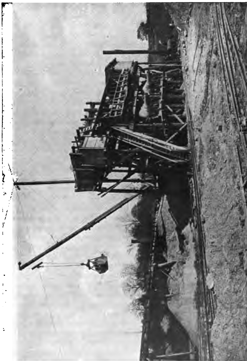
PLATE 170.—Central Concrete Mixing Plant of Large Capacity. Sand and stone raised to bins by derrick with "grab" bucket. Concrete mixed in tilting mixer which discharged into bottom-dumping buckets hauled to site of work on cars.
